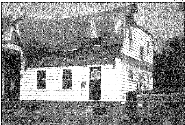
Donated to Cheshire Housing Trust by Keene State College, this house is shown in the process of being moved.
